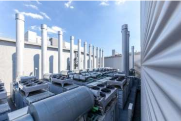
Data Centres E-Shelter, Germany Evoswitch, Netherlands Google, California
